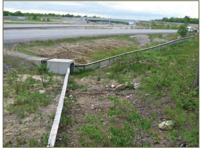
Photo 53. Fencing approaching tunnel entrance in a 'V' pattern © K. Gunson
