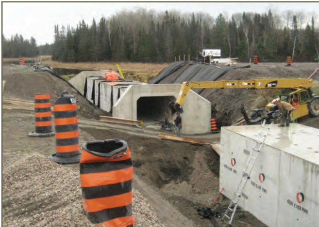
Photo 20. 3.4 x 2.4 m concrete box culvert connecting wetland habitat used by turtles on highway 69. © K. Gunson
