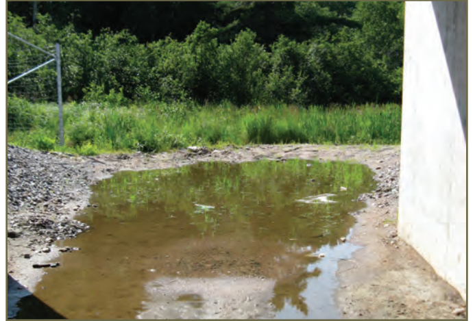
Photo 31. Water accumulation at tunnel entrance. © K. Gunson
