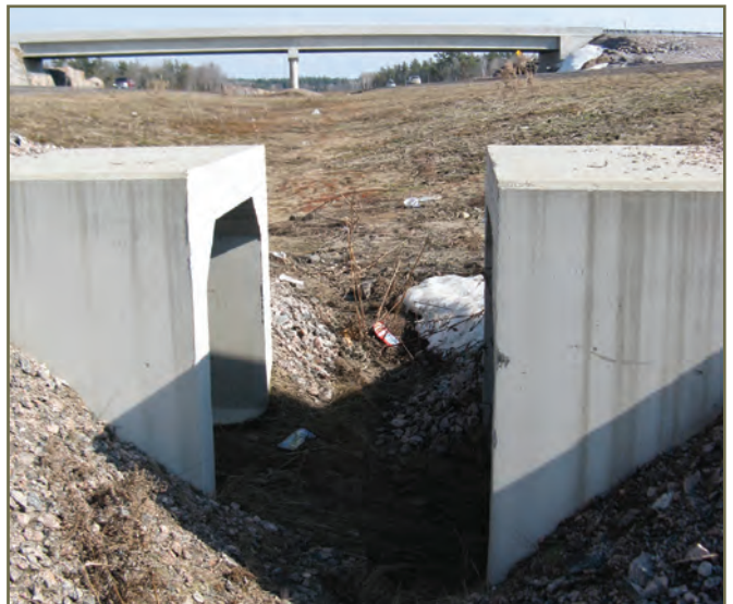
Photo 10. Box tunnels in median that should be connected with a fence when intended for wildlife passage. © K. Gunson
