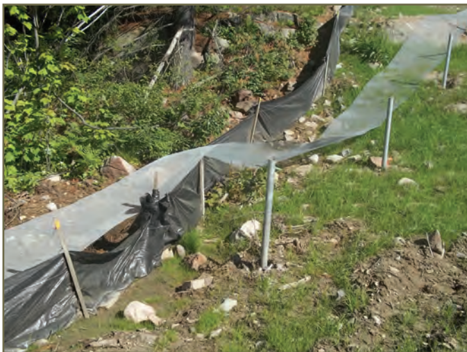
Photo 63. Temporary fencing installed prior to installation of more permanent fencing along highway 69, note permanent fencing completed in Photo 48. © W. Kowbasniuk
