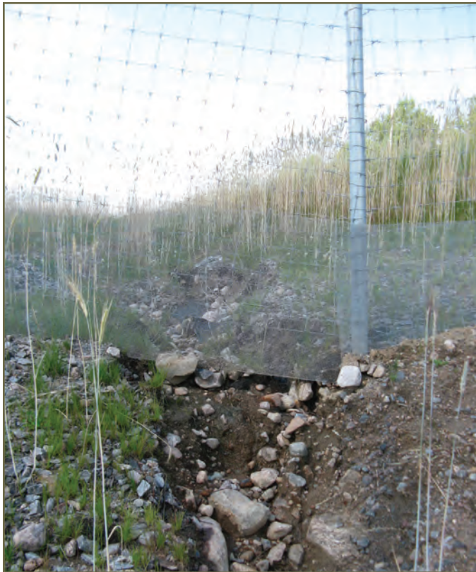
Photo 50. Fence with gap at bottom due to erosion from water draining under fence © K. Gunson
