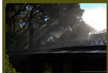
Photo 1. Roof mounted sprinkler.
