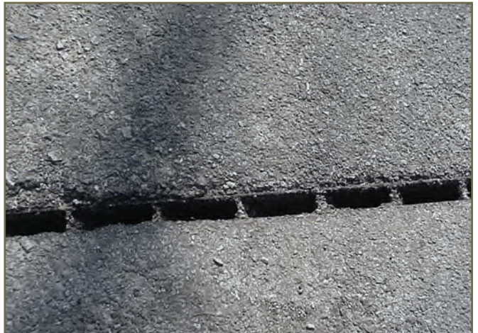
Photo 17. Zoom-in of open-top pipe culvert at road for Timber Rattlesnakes in Illinois, U.S. © S. Ballard
