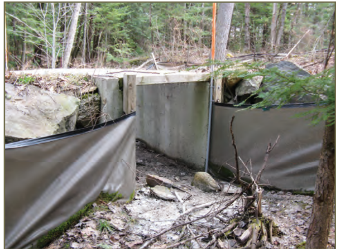
Photo 51. Fence tying into tunnel at Rice Lake Trail, Note shade cloth not recommended for permanent fencing © K. Gunson
